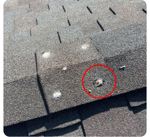
Exposed nail heads at ridge shingles.
