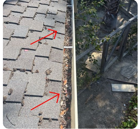
Debris accumulation within gutter system.
