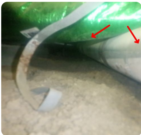
Water/silt lines at cooktop fan ducting.
