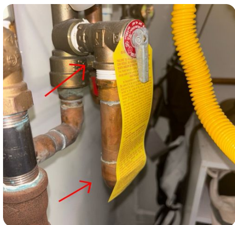
Water heater TPR valve with discharge tube.
