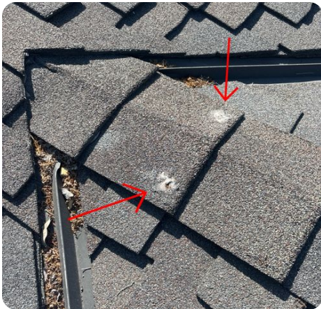
Exposed nail heads at ridge shingle.
