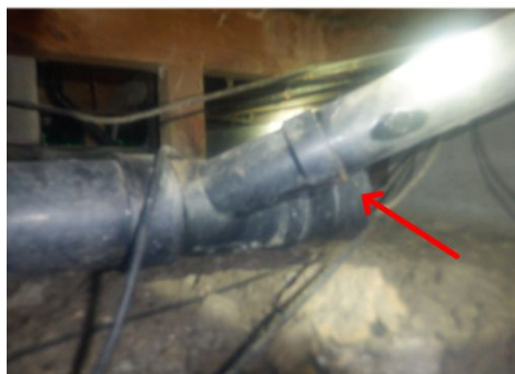
Leaking waste fitting below kitchen.
