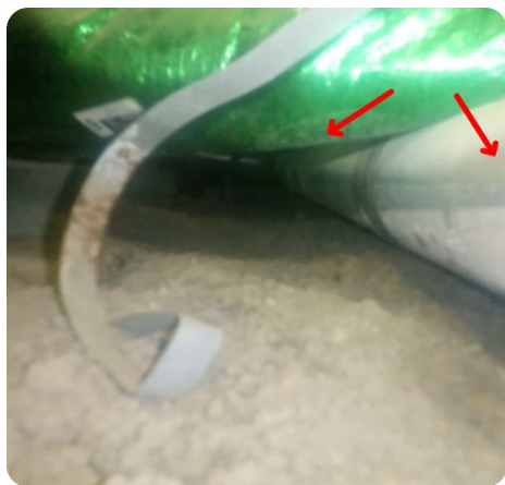
Water/silt lines at cooktop fan ducting.
