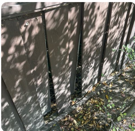
Unsecured boards at perimeter fence.
