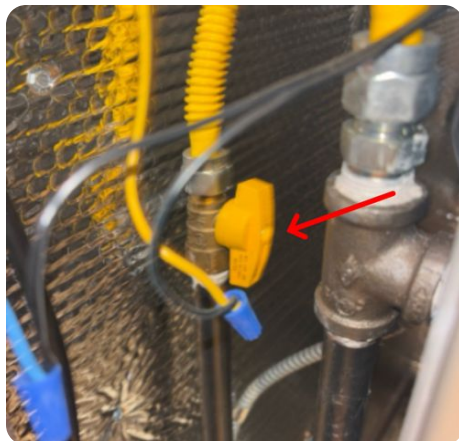
Natural gas control valve serving furnace.
