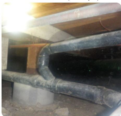
Functional ABS waste plumbing within crawl space.
