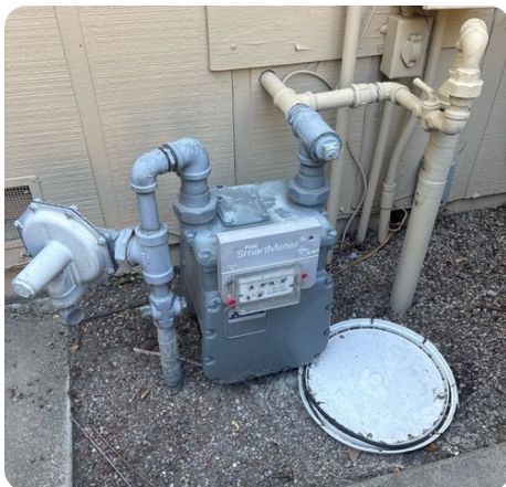
Natural gas meter at garage exterior.
