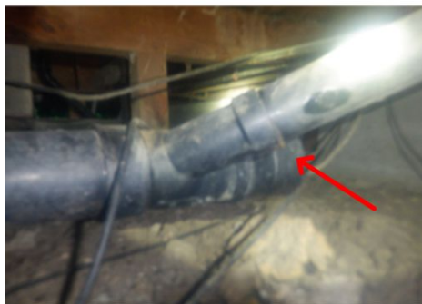
Leaking waste fitting below kitchen.
