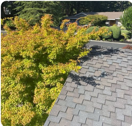
Tree overhanging garage roof surface.
