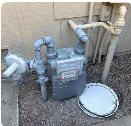
Natural gas meter at garage exterior.
