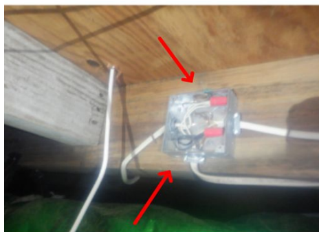
Open junction box within crawl space below bedroom 2.
