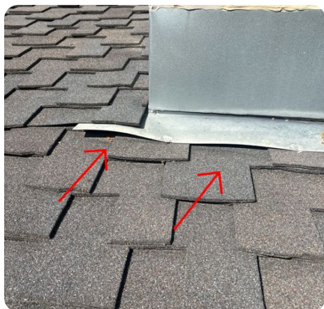
Lifting flashing at base of chimney structure.
