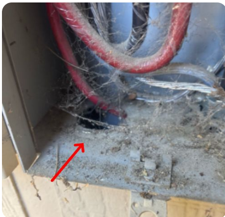
Knock-out lacks a bushing at base of main panel .
