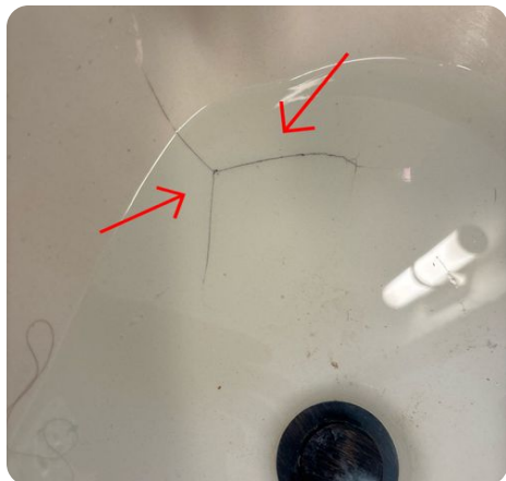
Cracked master bathroom basin.
