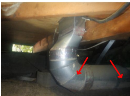
Water/silt lines at cooktop fan ducting.
