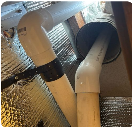
Functional furnace exhaust flue.
