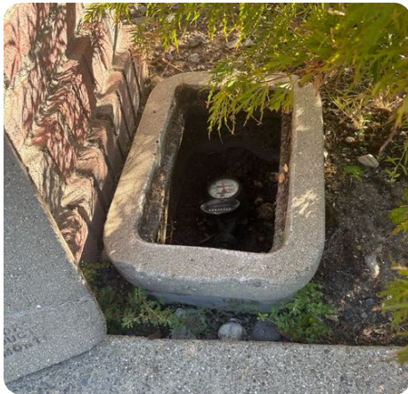
Water meter in landscaping strip adjacent to curb.
