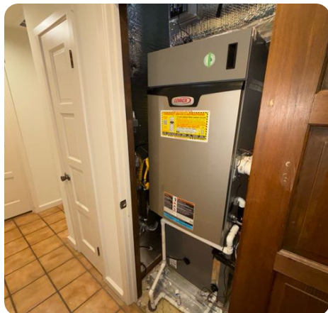
Lennox branded, high efficiency, natural gas furnace within hall utility closet
