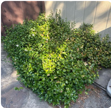
Vegetation in contact with exterior siding material.
