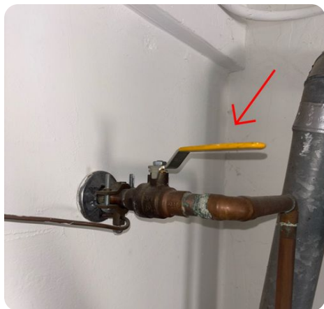
Cold water supply valve serving water heater.
