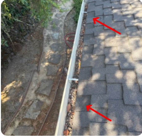
Debris accumulation within gutter system.
