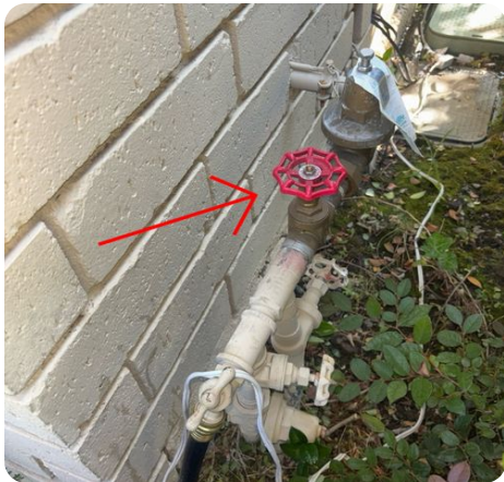
Main water control valve at garage exterior.
