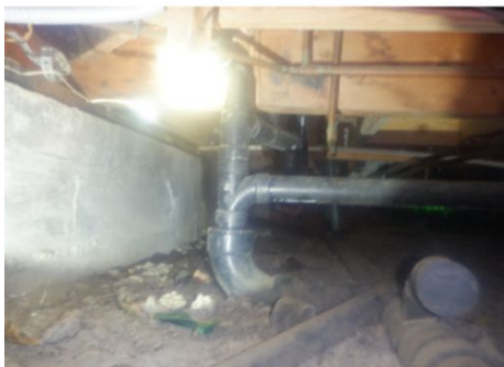
Functional ABS waste plumbing within crawl space.
