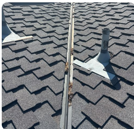
Debris accumulation at roof surface.
