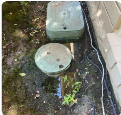
Trapped standing water at landscaping adjacent to garage exterior.
