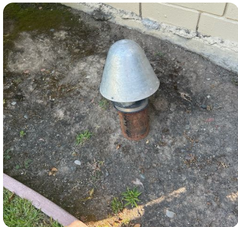
Sewer clean-out at front of home.
