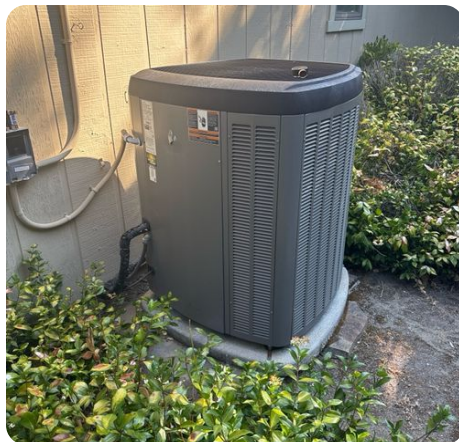
Lennox branded condensing unit at hall bathroom exterior.
