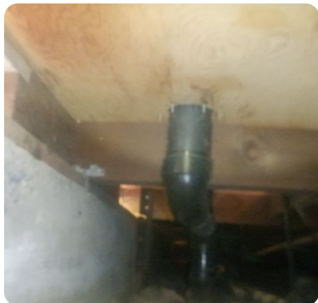
Functional ABS waste plumbing within crawl space.
