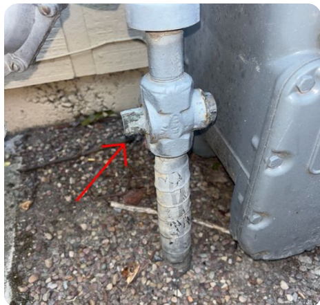
Natural gas control valve at meter riser.
