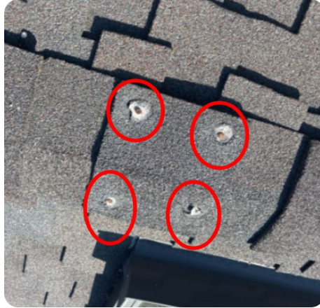
Exposed nail heads at ridge shingles.
