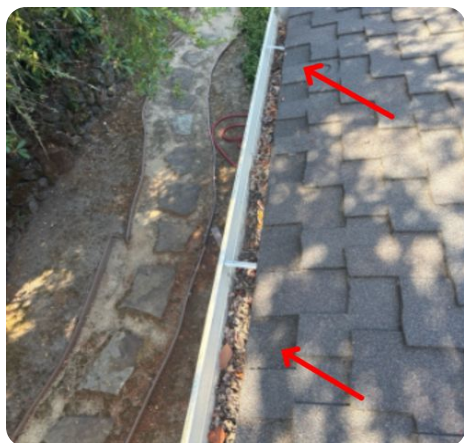
Debris accumulation within gutter system.
