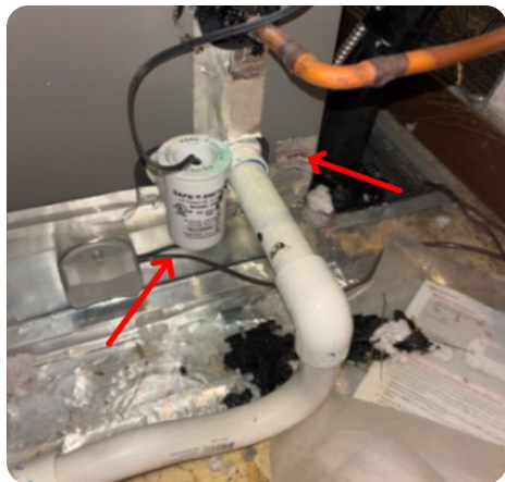
HVAC condensate drain line with safety switch serving evaporation coil.
