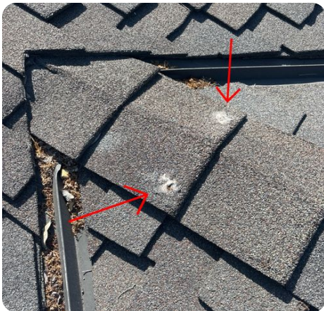
Exposed nail heads at ridge shingle.
