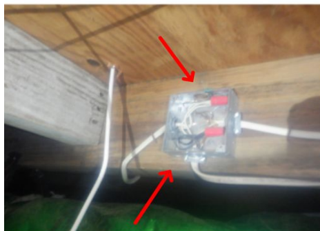
Open junction box within crawl space below bedroom 2.
