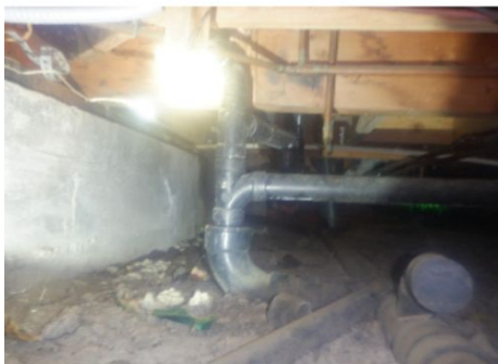
Functional ABS waste plumbing within crawl space.
