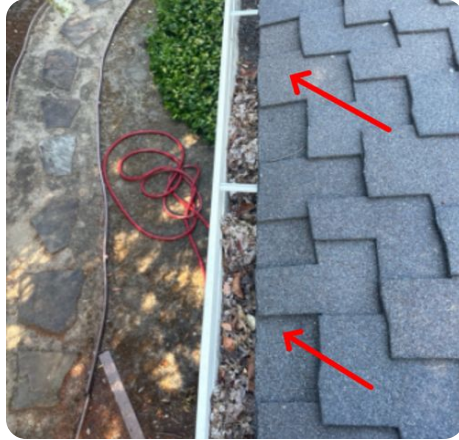
Debris accumulation within gutter system.
