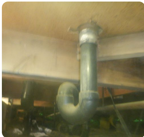
Functional ABS waste plumbing within crawl space.
