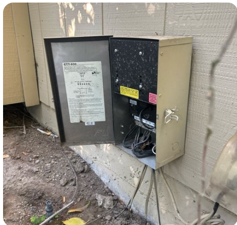
Low-voltage transformer at bonus room exterior.
