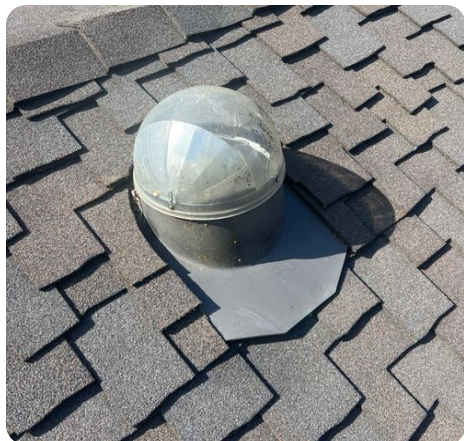
Functional tubular skylight as viewed from roof surface.
