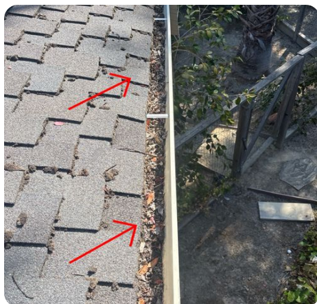
Debris accumulation within gutter system.
