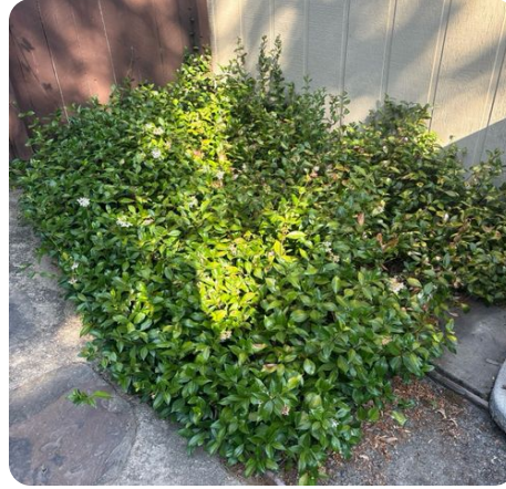
Vegetation in contact with exterior siding material.
