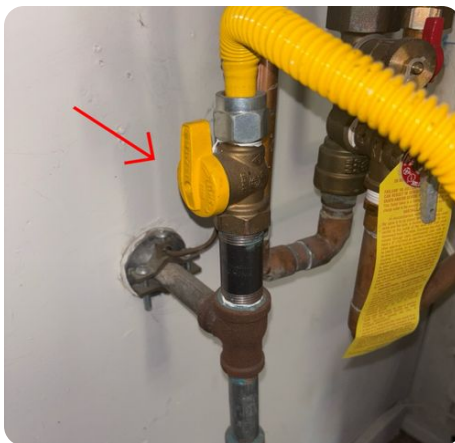
Natural gas control valve serving water heater.
