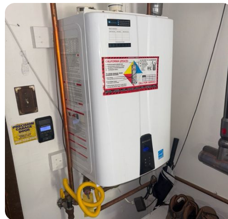
Navien branded, high efficiency, tankless natural gas water heater within garage
