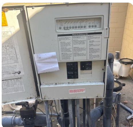
Auxiliary service panel supporting pool equipment.
