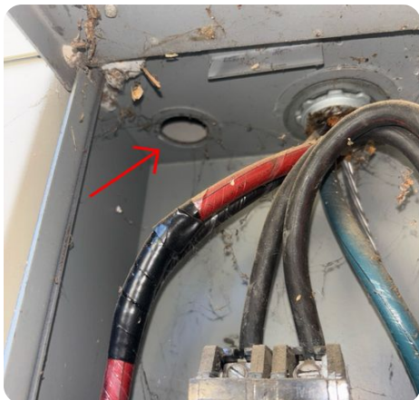
Open knockout at top of main service panel.
