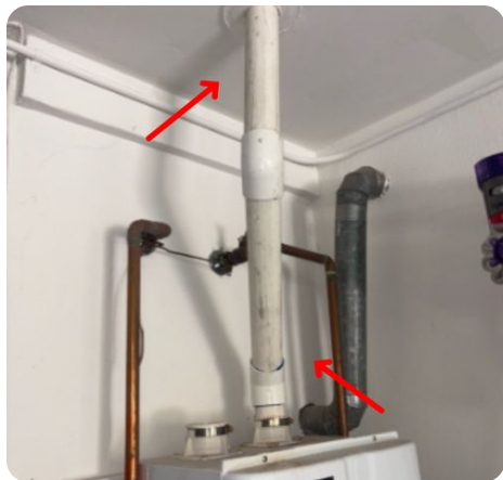
Functional water heater exhaust flue.
