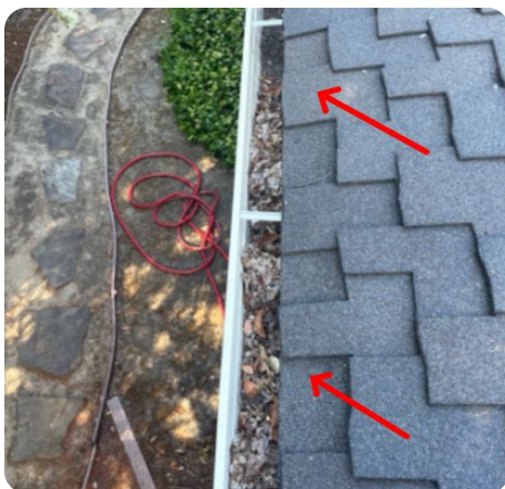
Debris accumulation within gutter system.
