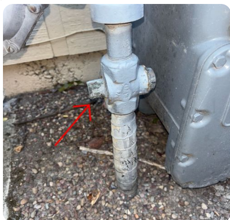
Natural gas control valve at meter riser.
