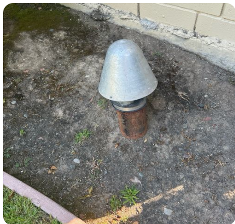
Sewer clean-out at front of home.
