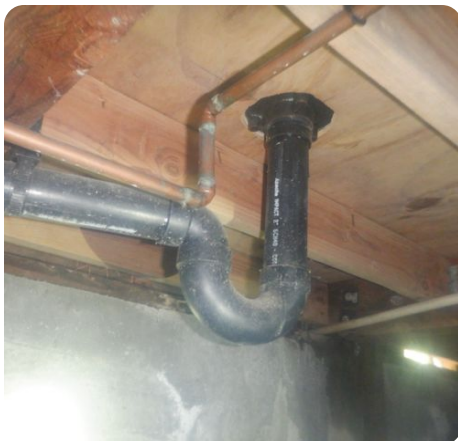
Functional ABS waste plumbing within crawl space.
