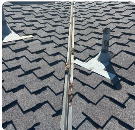
Debris accumulation at roof surface.
