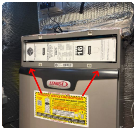
Clean disposable HVAC filter at enclosure above furnace.
