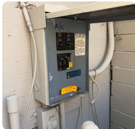
Supplemental sub-panel at garage exterior.
