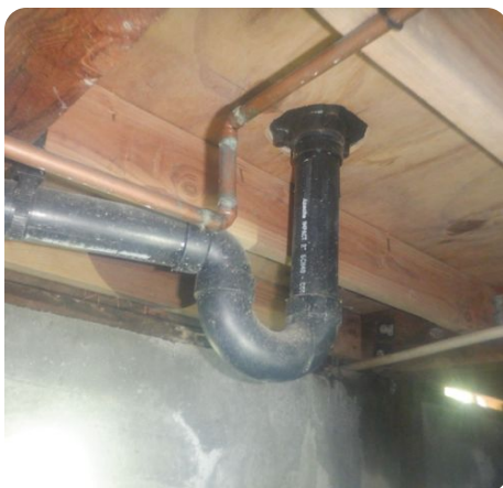
Functional ABS waste plumbing within crawl space.
