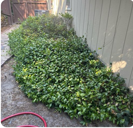
Vegetation in contact with exterior siding material.
