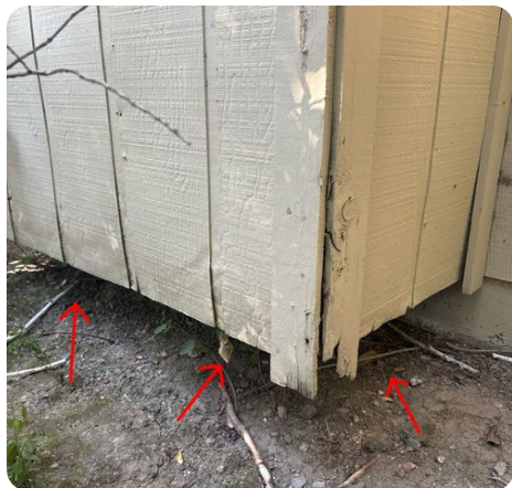
Moisture related damage at exterior siding and trim serving fireplace chase.
