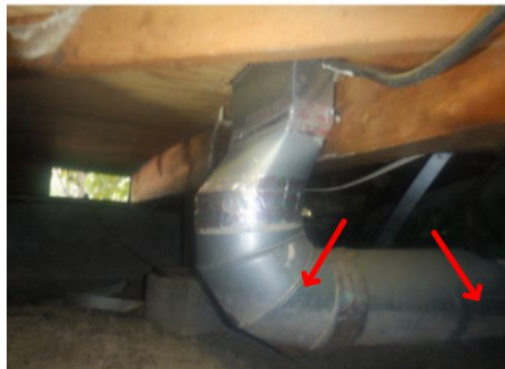
Water/silt lines at cooktop fan ducting.
