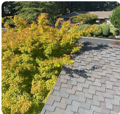
Tree overhanging garage roof surface.
