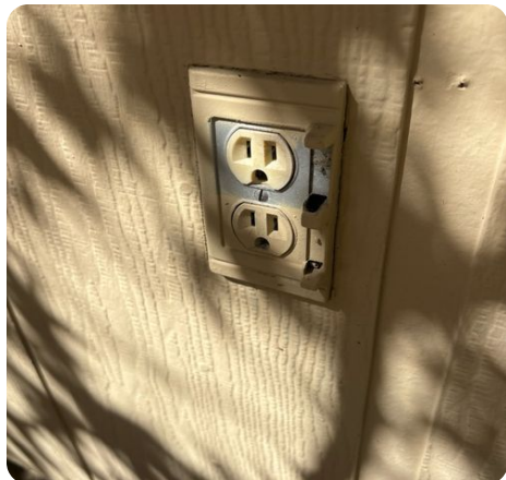
Damaged weatherproof outlet cover at rear of home.
