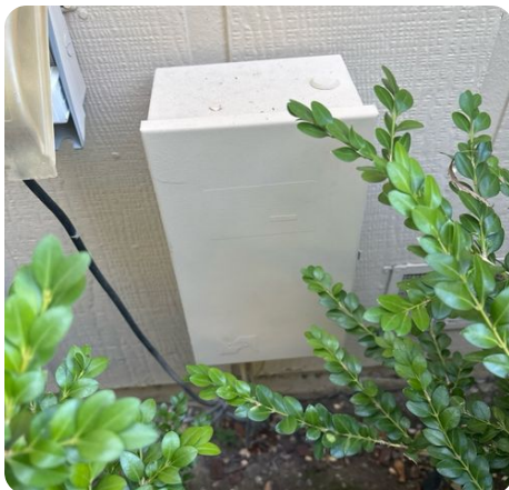
Low-voltage transformer at family room exterior.
