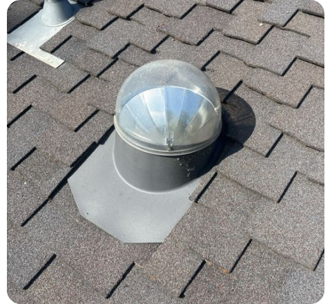
Functional tubular skylight as viewed from roof surface.
