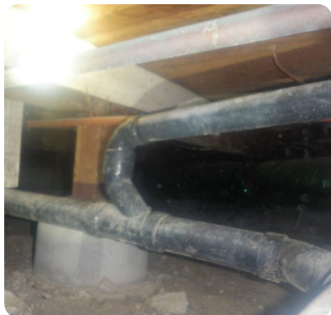
Functional ABS waste plumbing within crawl space.
