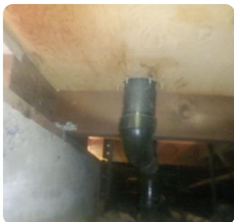
Functional ABS waste plumbing within crawl space.
