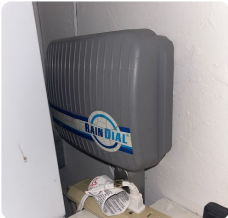
Irrigation control module within garage.
