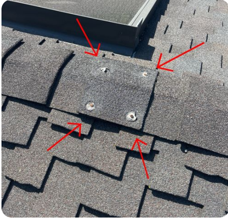
Exposed nail heads at ridge cap.
