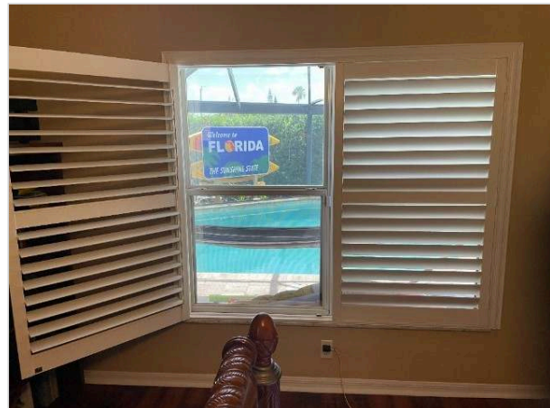
Affected primary bedroom window.
