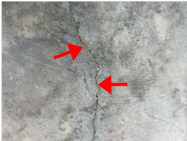
Minor crack in garage floor.
