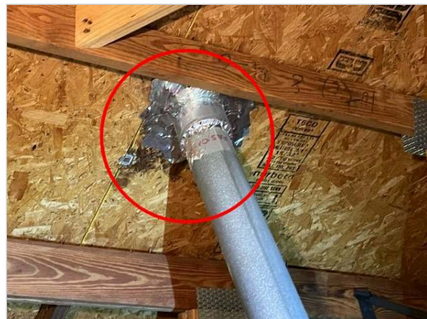
Past stain and repair.
