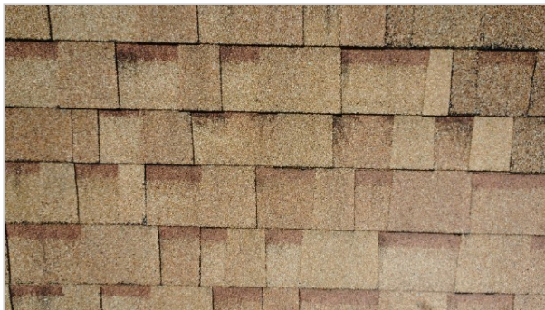
Roof cover greater than 15 years per posted permits.
