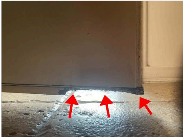
Damaged weather strip on bottom of door.
