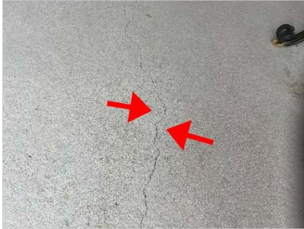
Minor crack in front porch slab.
