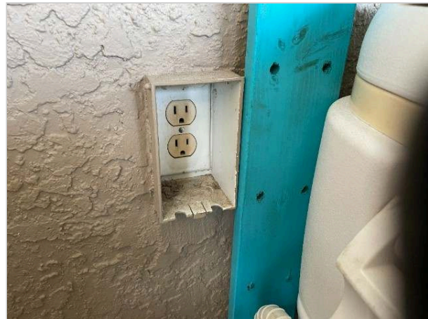
Exterior outlet cover missing in back.
