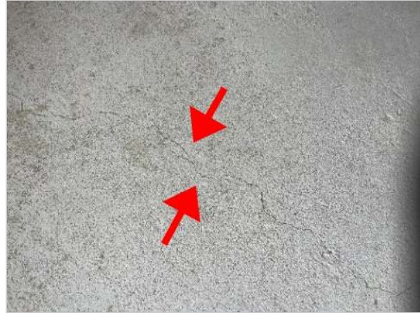
Minor crack in front porch slab.
