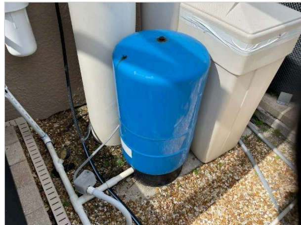
Well expansion tank.
