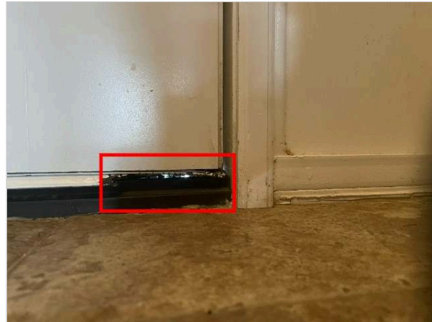
Gap at damaged weather strip.
