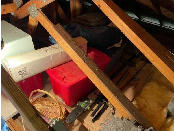
Stored items over the garage.
