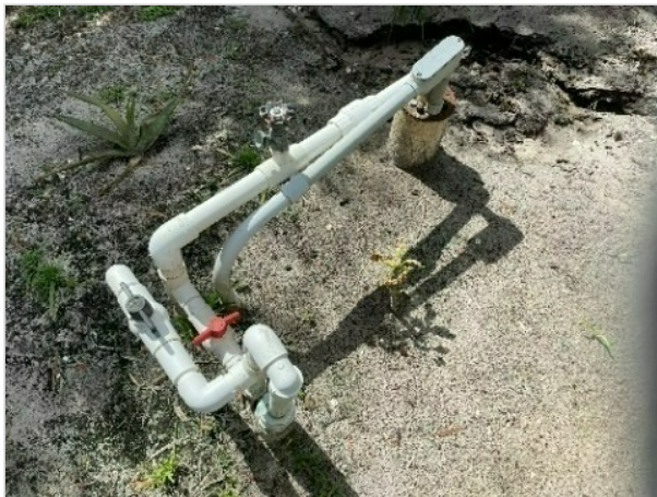
Well head and plumbing.
