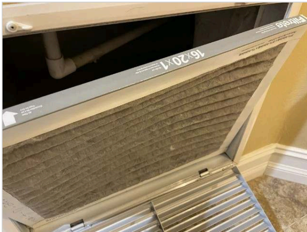
Filter is dirty.
