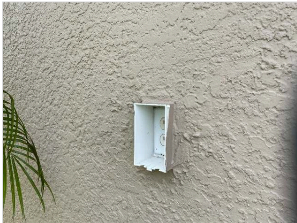
Exterior outlet cover missing on North side.
