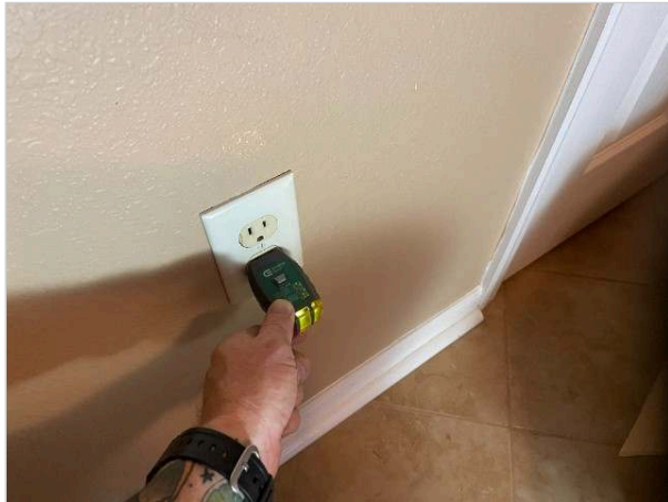
Loose outlet in primary bedroom West wall.
