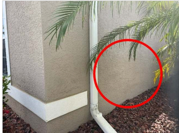
Affected area on South side.
