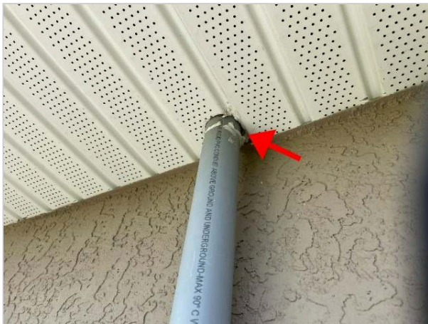
Penetration needs re-sealed on South side.
